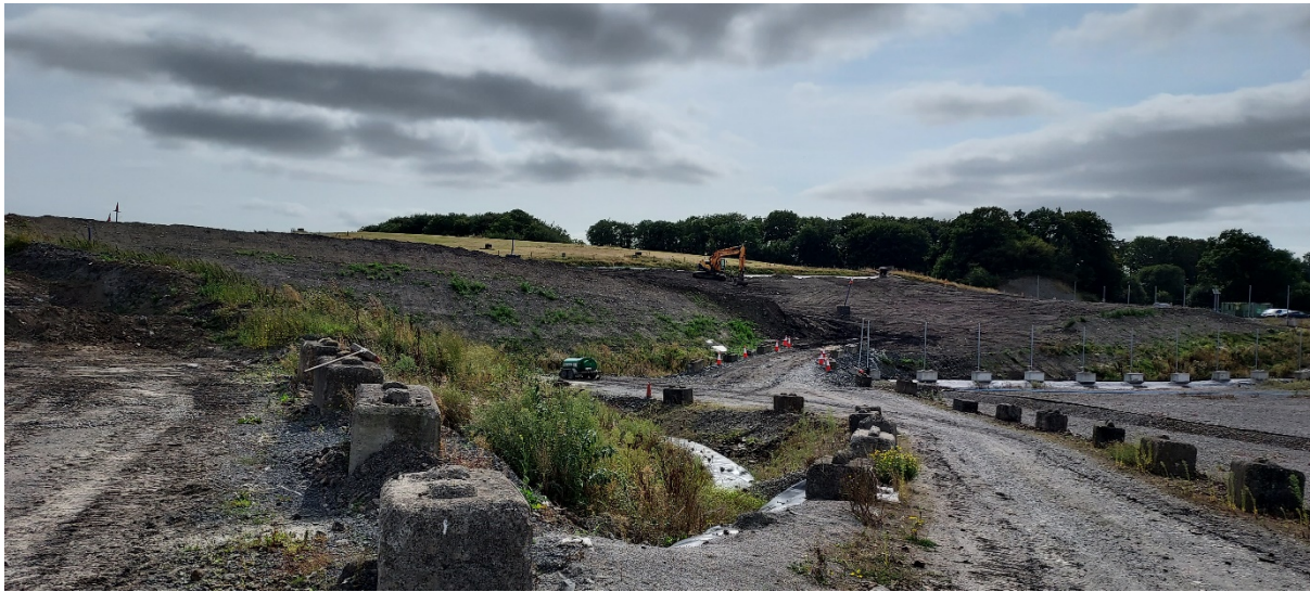
Ballaghveny landfill - view from the top of the ramp down to the waste tipping face in Cell 10B
