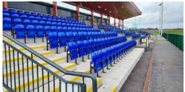
Fethard Town Park completed the installation of 400 spectator seats with a grant contribution of €32,000.
