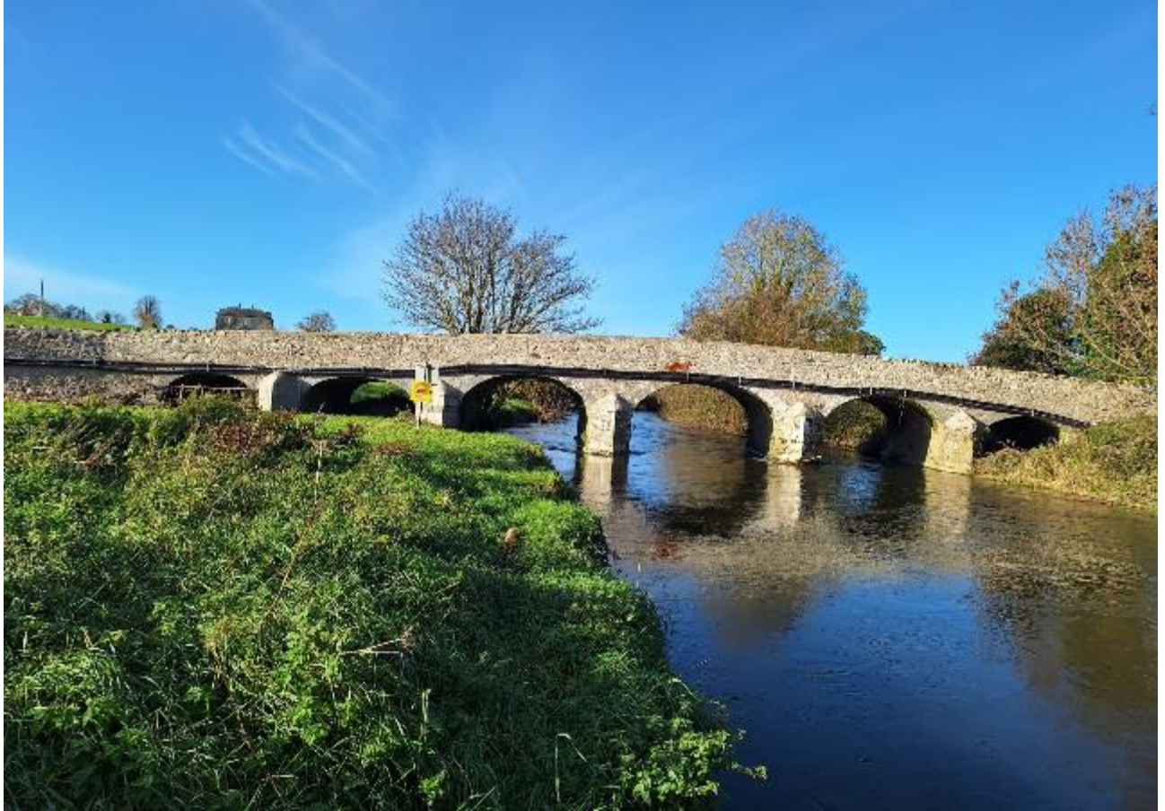
Annaghbeg Bridge – Seven-Arch Masonry Bridge spanning the Nenagh River completely restored. The Bridge is a Protected Structure and was built sometime in the 1750's.
