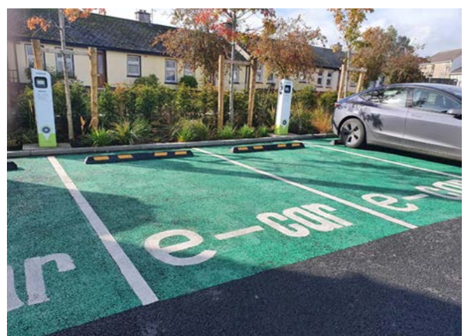
EV Chargers installed in John's Lane Car Park, Nenagh, by Tipperary County Council
