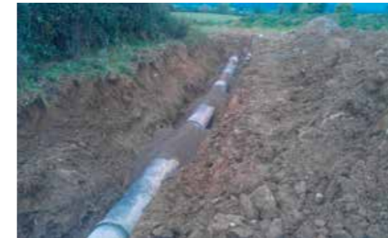
Pipeline on the Thurles Regional Water Supply Scheme
