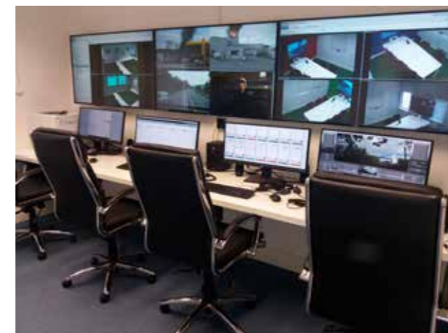
Clonmel 'HYDRA' Suite - Control Room
