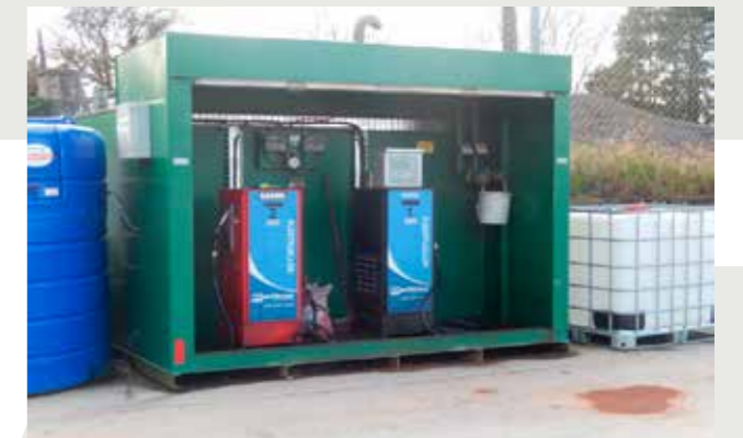
Self contained and banded fuel storage tanks and dispensing system
