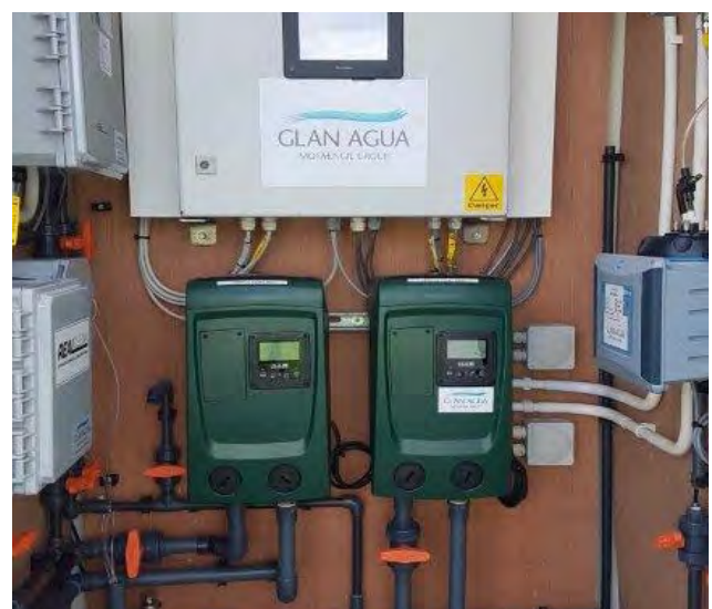
Borrisokane Water treatment plant ultra violet water filter June 2021
