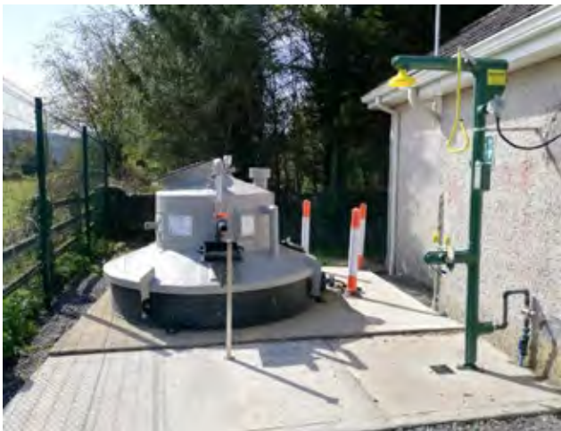
Cordangan, Tipperary water treatment plant chlorine dosing
