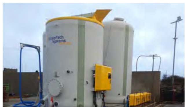
Brine Saturator, installed at Waller's Lot, Cashel
