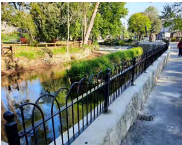
Newly restored stone wall and new bow top railing that was installed as part of the works
