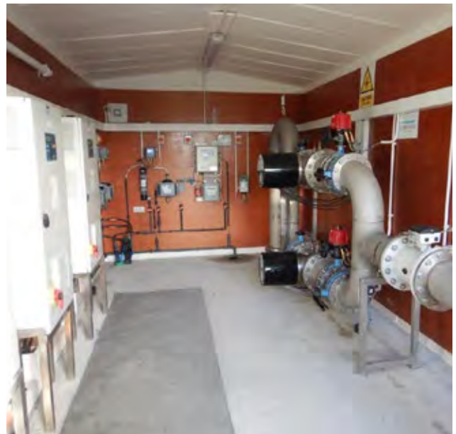
Monroe, Clonmel water treatment plant disinfection upgrade
