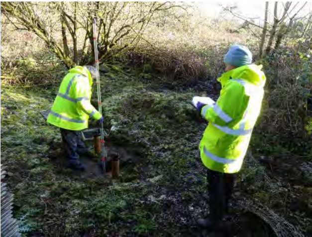
Figure 2 Septic Tank Inspection: Staff from the Environment and Climate Action Section (Fergus O'Connor, Executive Engineer, and Paula O'Dwyer, Executive Scientist) determining the level of sludge in the tank using "The Sludge Judge".
