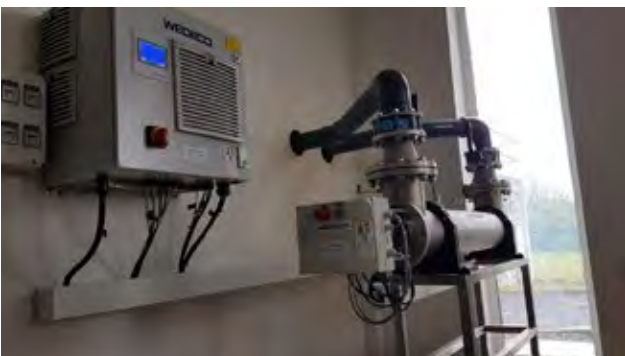
Borrisokane water treatment plant ultra violet water filter June 2021
