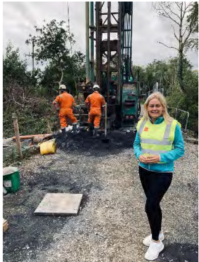
Figure 1. Ardcrone Group Water Scheme Manager, Eleanor Maher, and Fogarty Well Drilling Ltd., personnel at the Production Well at Mountfalcon, Borrisokane.
