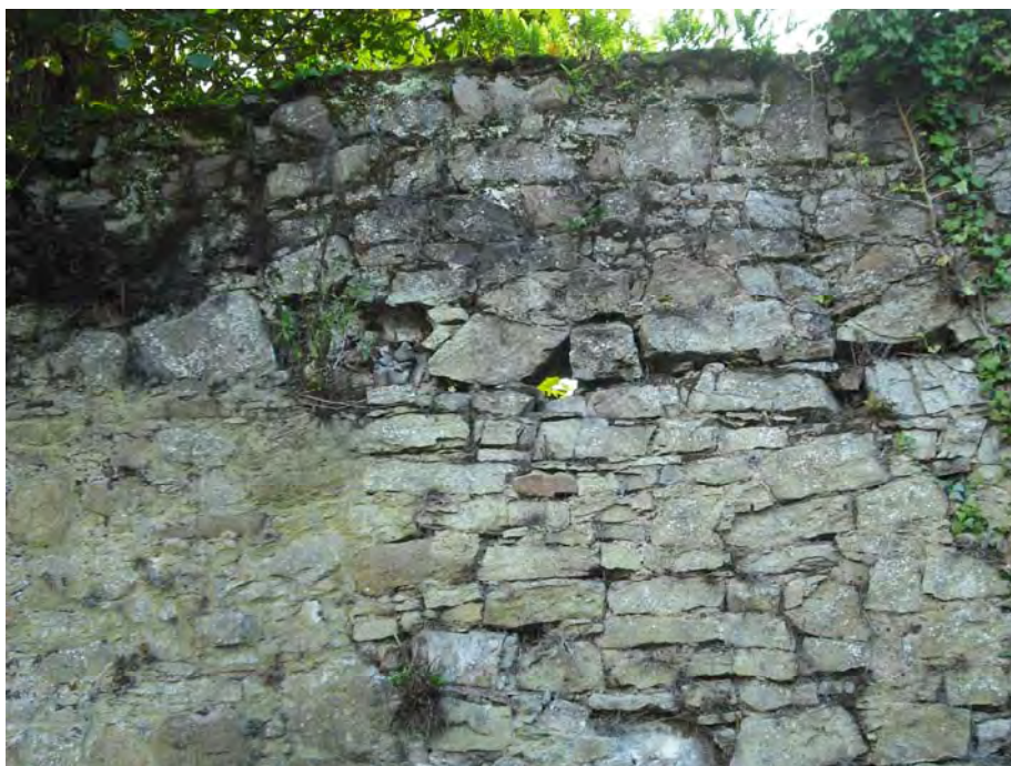
Picture 6 Void in Wall A (top 1.5m unstable)
