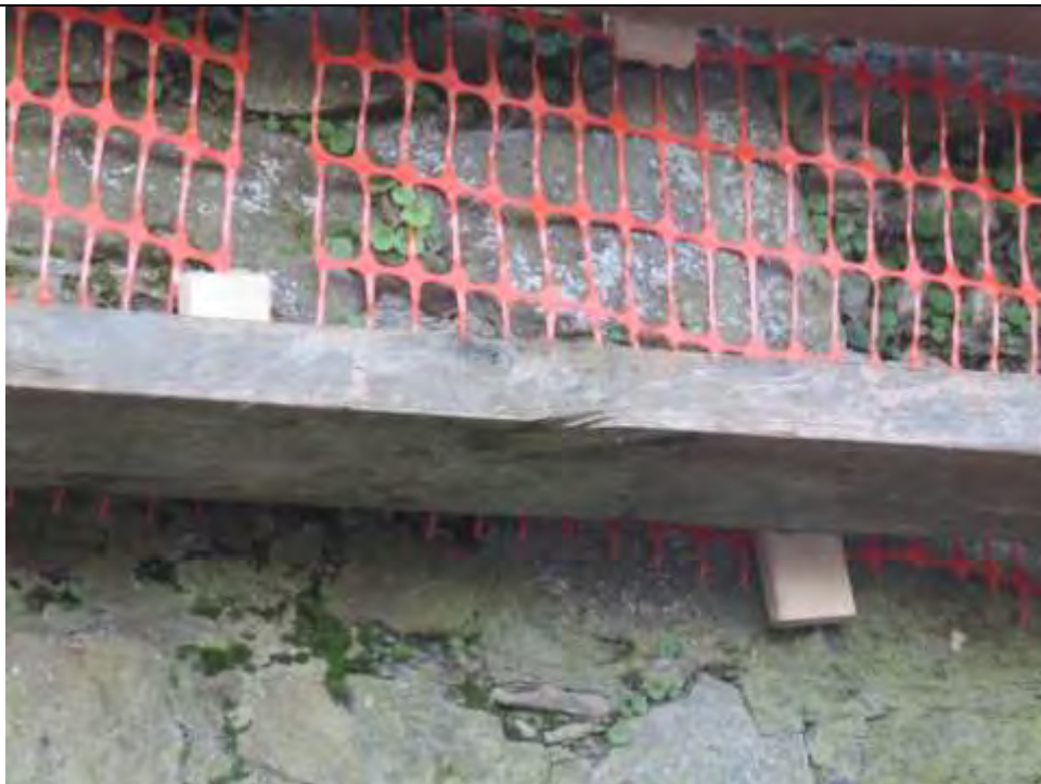
Fig. 24) The top of the wall was covered with an open plastic netting to catch any falling stones and to allow the wall air movement - this picture also shows the wedges in place.
