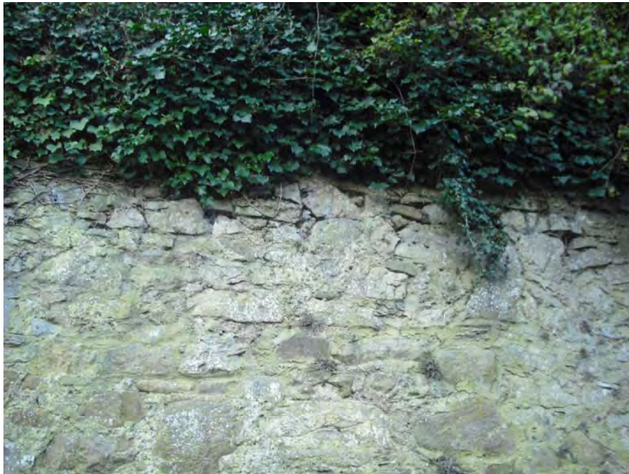
Picture 1 Open Masonry Joints High Level Wall A
