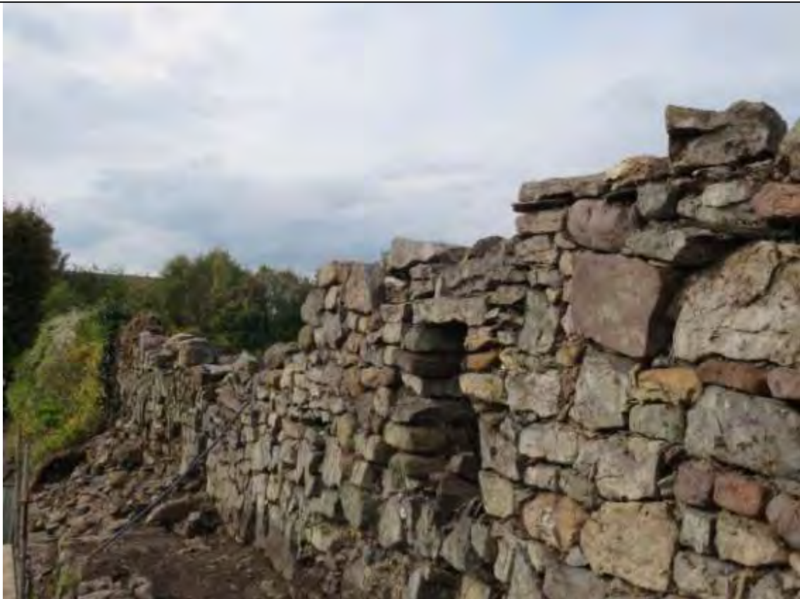
Fig. 15) A section of a previous ope now blocked up.
