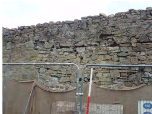
Plate 16. Horizontal breach along walkway parapet, external, north wall.
