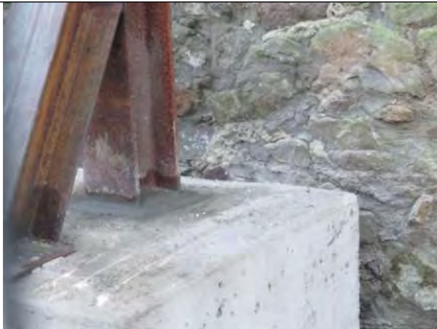
Fig. 22) When all timbers and brackets were in place the main steel stanchion was grouted up.
