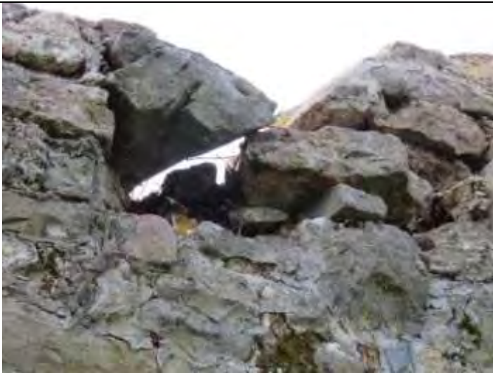
Fig. 14) Precarious masonry just resting there.
