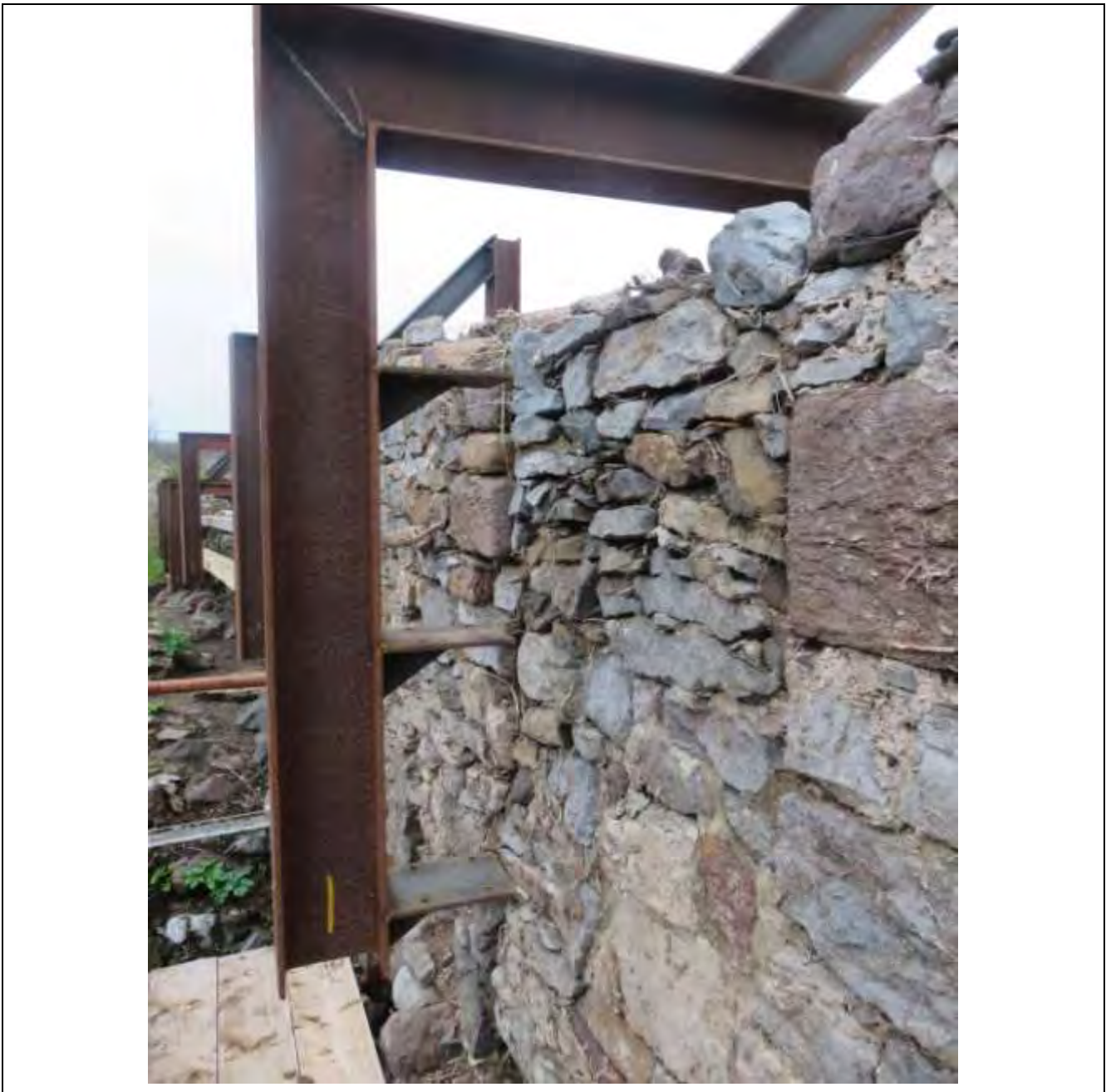
Fig. 18) The metal beams wrap over the wall to give support to the south elevation
