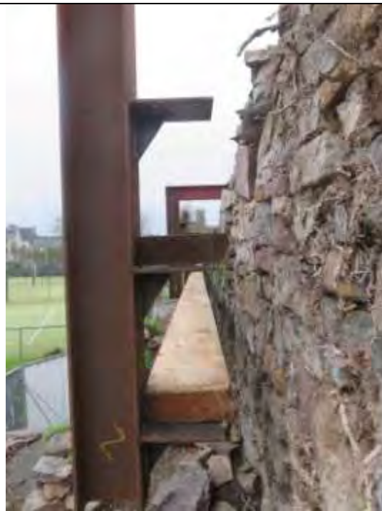
Fig. 19) With the timber rails which then will be wedged to the wall.
