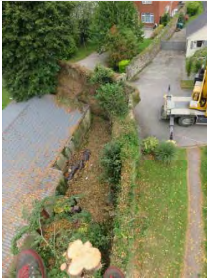
Fig. 8) A view from the boson's chair of the section of the wall treated in 2014.
