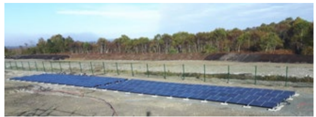
Solar PV panels installed at Ballaghveny Landfill
