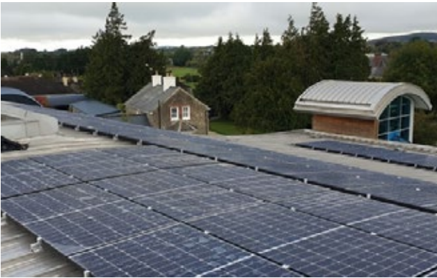
PV panels on the roof of Roscrea Leisure Centre
