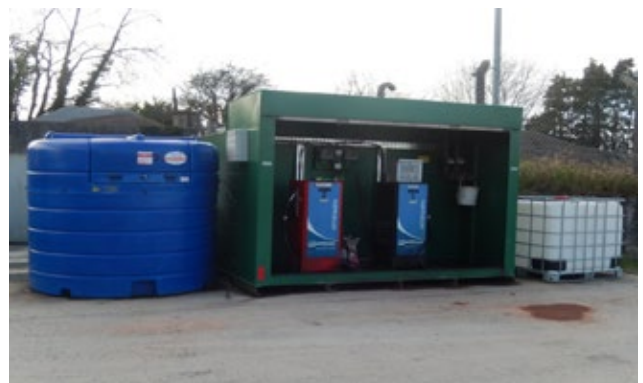
Automated Diesel Fuel and Adblue Dispensing System
