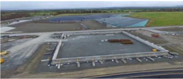
2020 Bunded area for new leachate tank under construction (in the foreground) and landfill empty lined cells (in the background)
